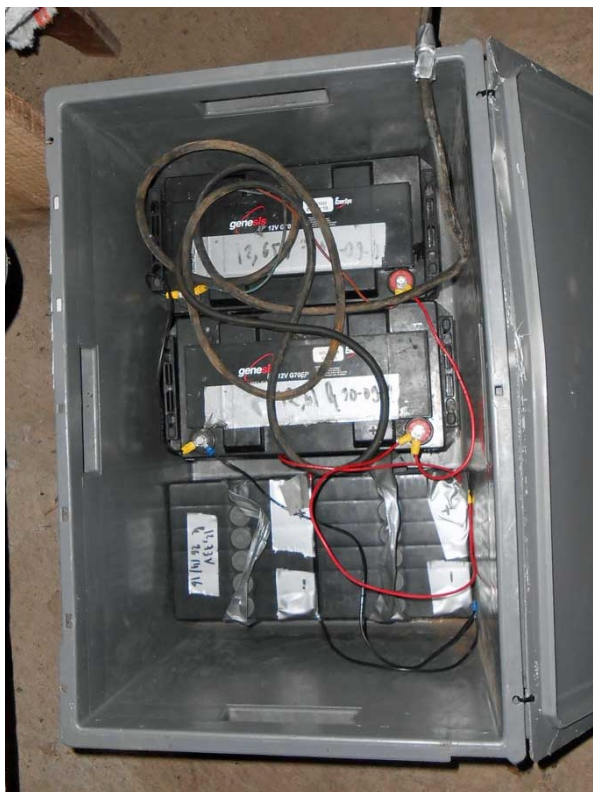
Caisses batteries 12V
